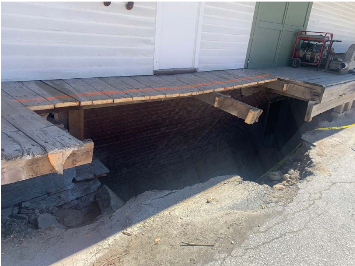
4/24/2026: West River Street drainage issue closeup
